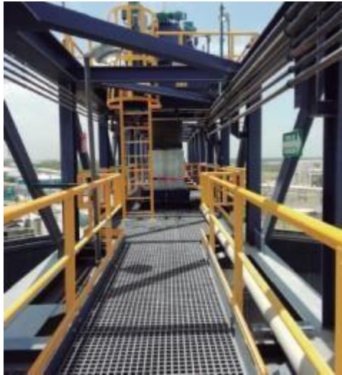
PUENTE TANQUE SETTLER 60%
